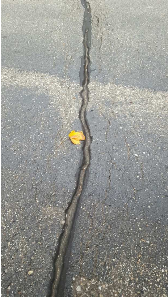
Crack not filled to top
