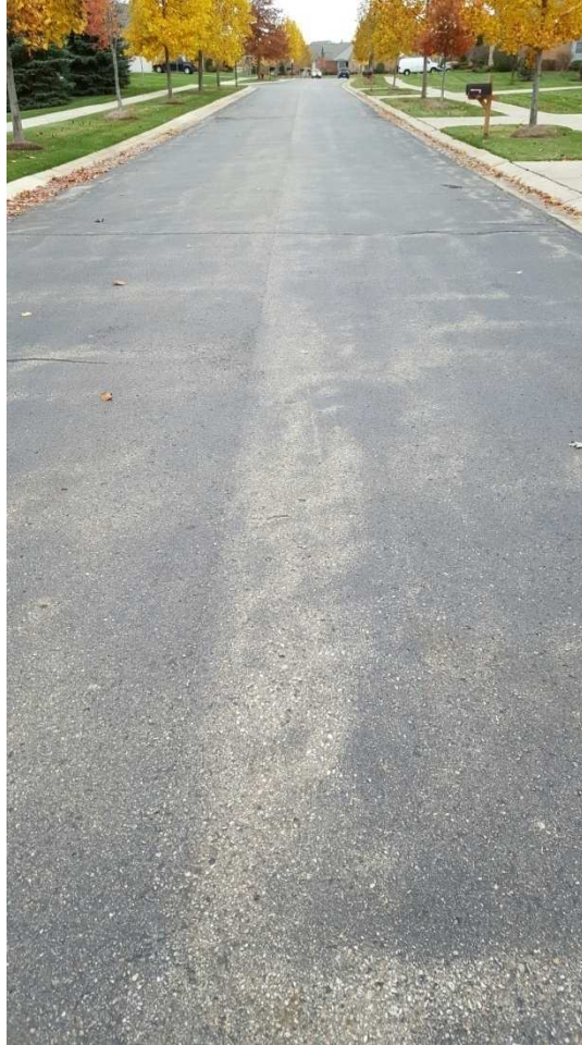
Surface not well covered or uniform
